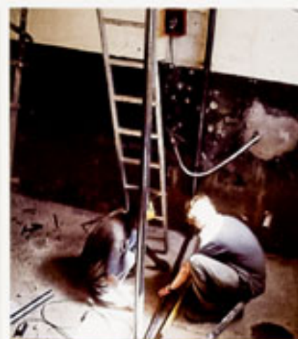
Mark and Joseph measuring and welding the steel bars that would eventually separate the enclosure into two.
