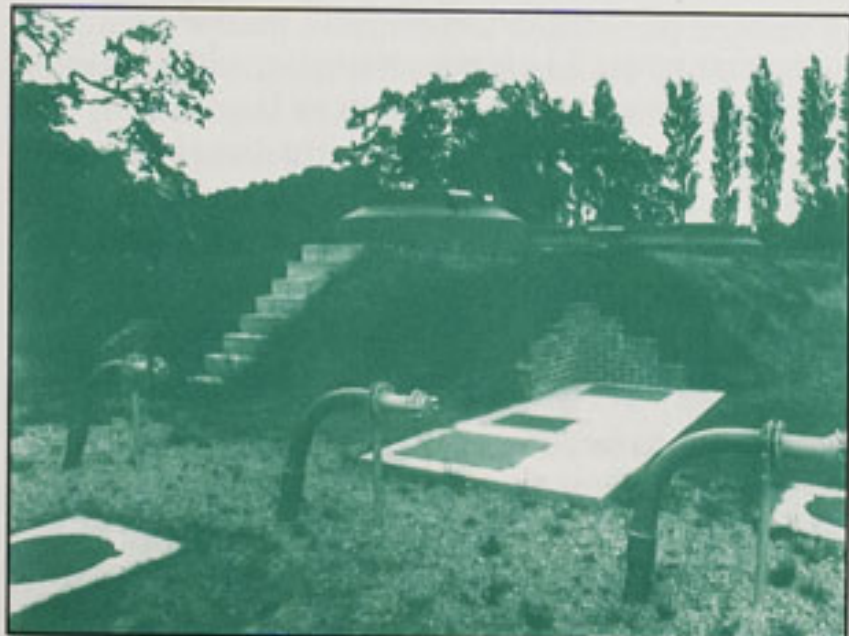
New sewerage treatment plant installed to meet NRA environmental standards.
