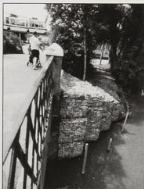
Neat gabion work saved the foundations of the important bridge over the canal
